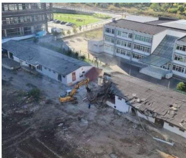
Fig. 3 In "Lakrishte" several NPB buildings are destroyed
